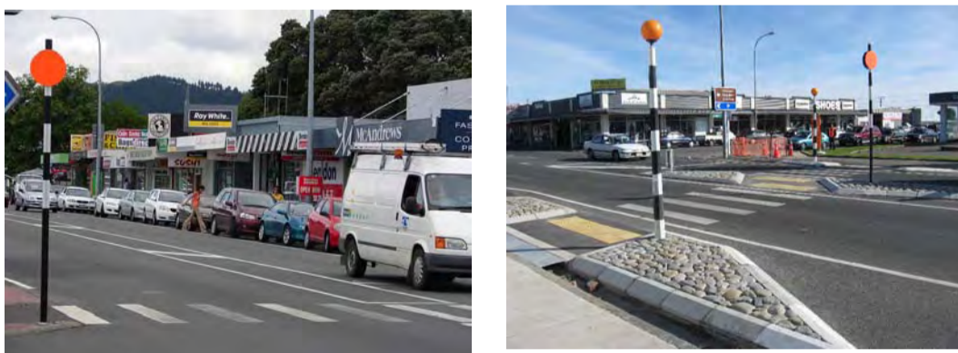
Figure 5. Before and after image of Otaki crossing improvements. River boulder finish matches with other similar features in the community.
